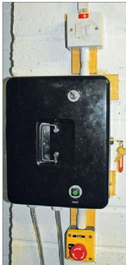
Photo 8. Inverter wall mounted control box.
